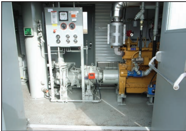
■ The gas compression package has been designed with ample room to operate and maintain the equipment. An FW Murphy control panel has been installed to monitor the operation of the package. The skid is equipped with heaters and an insulated building for cold weather operation.
